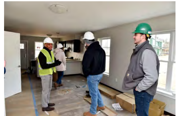
Keith Fairey, left, president and CEO of Way Finders, talks with members of his team in December in a unit under construction at their new project in Agawam, Rosewood Way Townhomes. (Don Treeger / The Republican)
